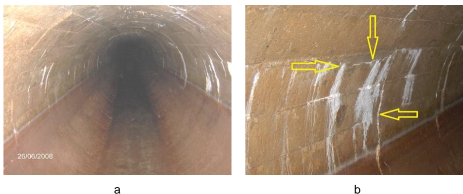
Fig. 3 Structural degradation of Strunga hydro-technical gallery located on AdII Timișești - Iași water supply pipe due to the site's ground pollutant effect; a - reinforced concrete water flow section; b - fissures and micro-fissures in the gallery wall (Luca et al. , 2008)
